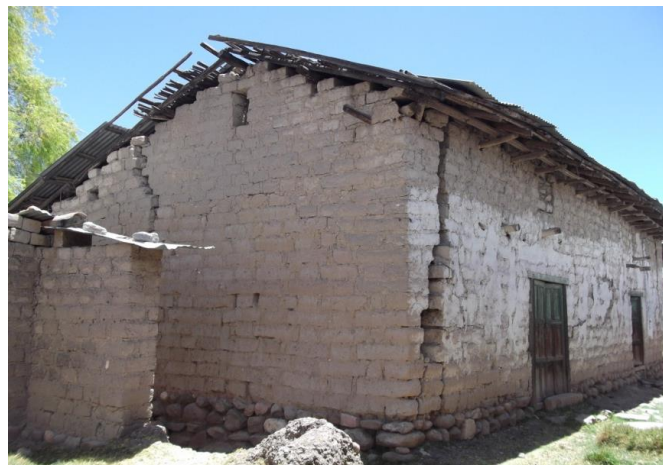
Figure 2. Inhabited damaged adobe house.
